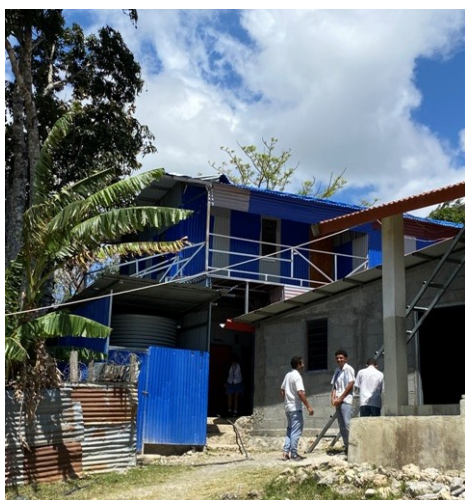
The new classroom built by the students above the toilets funded by Timbertop.
